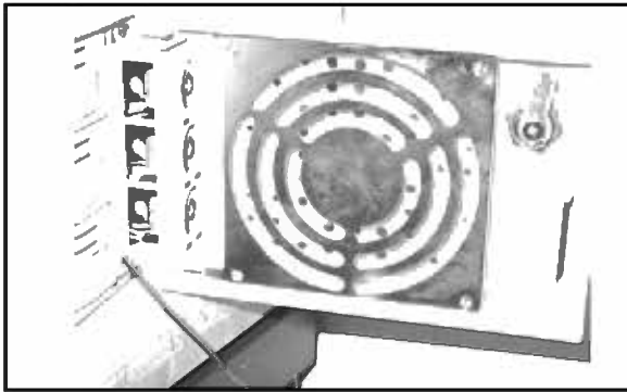
Figure 4.4 Noisy Backplane Fan Replacement
