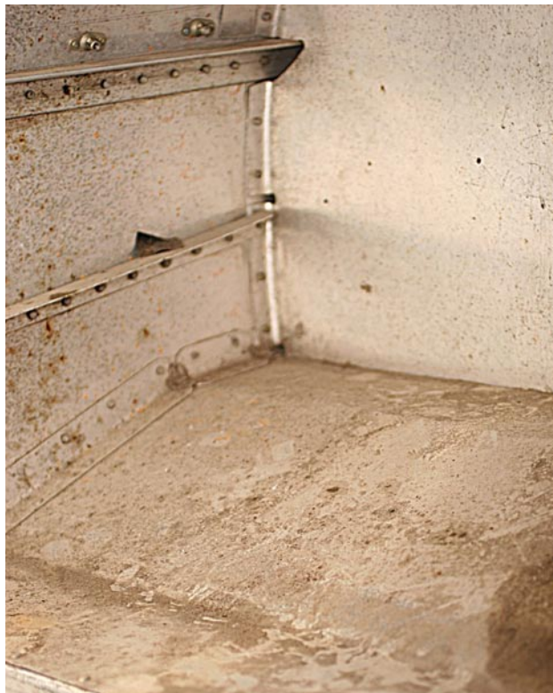
Figure 6-2. Direct chemical attack in a battery compartment.
