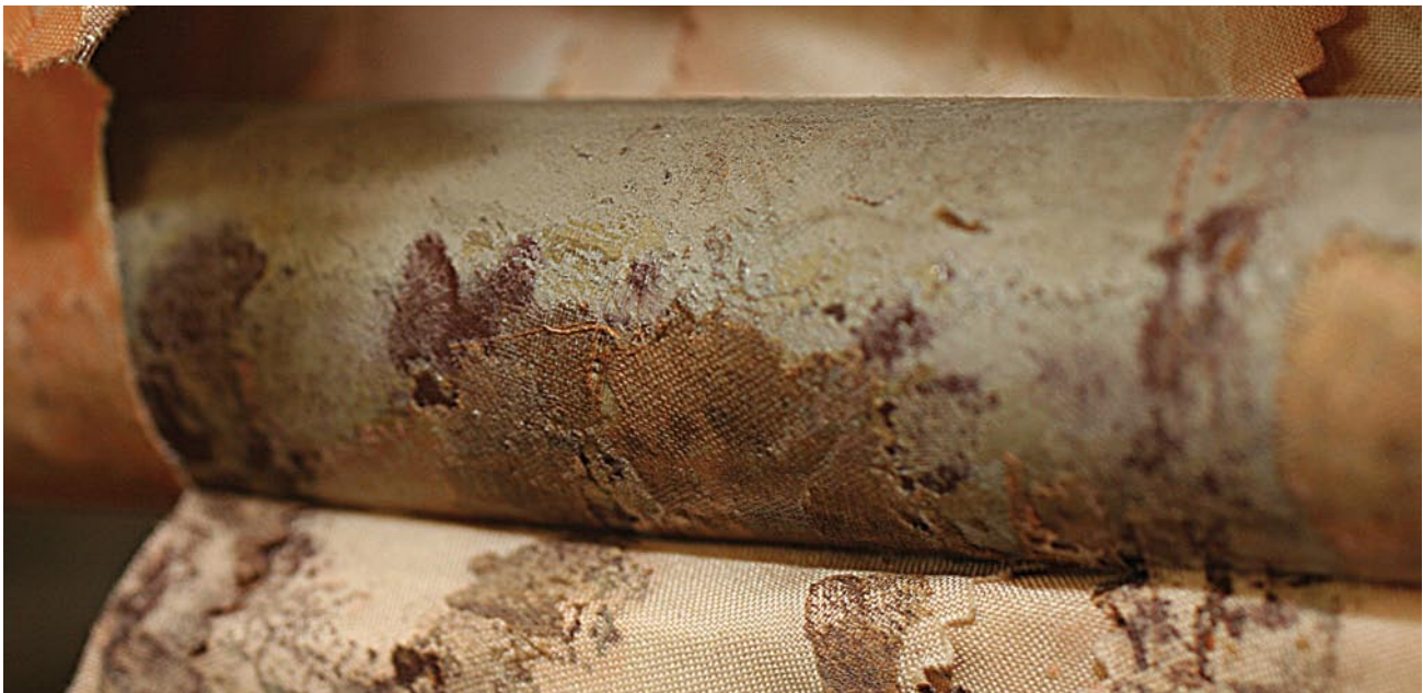
Figure 6-15. Rust on structural components.
