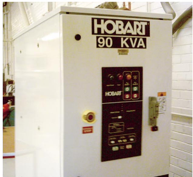
Figure 11-28. A stationary electrical power unit.
