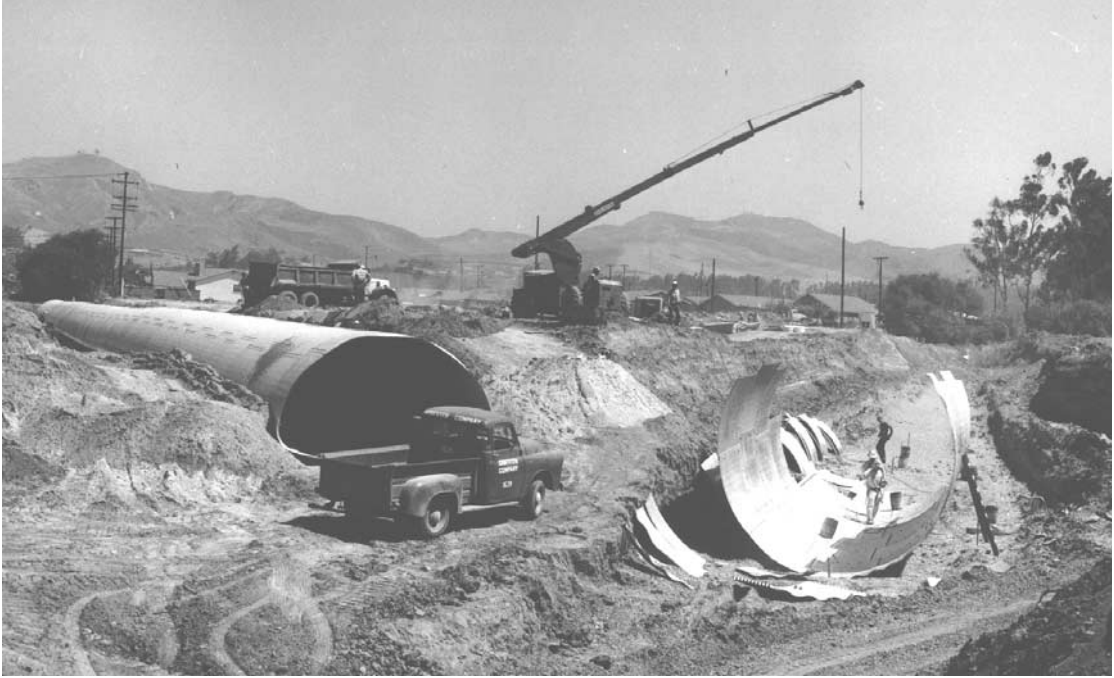
Fig. 10.21 Structural-plate pipe is shown being bolted together at right. Completely assembled structural-plate pipe arch is shown at left.
