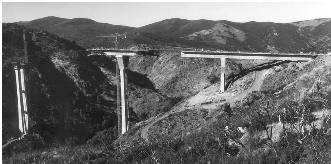
Fig. 17.54 Segmental cast-in-place concrete construction in progress for the Pine Valley Bridge, California. (California Department of Transportation.)
