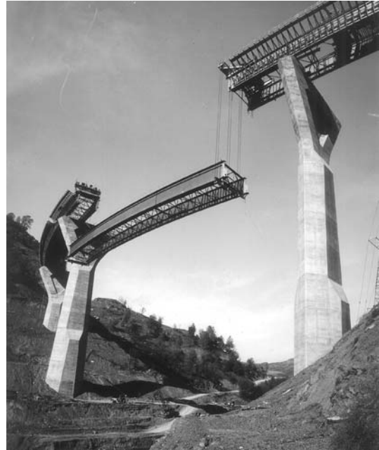
Fig. 17.33 Curved girders of Tuolumne River Bridge, California, were erected in pairs with their cross frames connected between them. (California Department of Transportation.)
