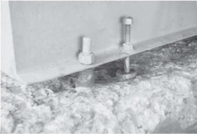
Figure 3-21: Manipulation of jack bolts and anchor bolts can re-shape equipment mounting surfaces
