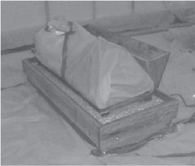
Figure 3-24: Grout forms are constructed to contain the grout. Note protective plastic on pump set
