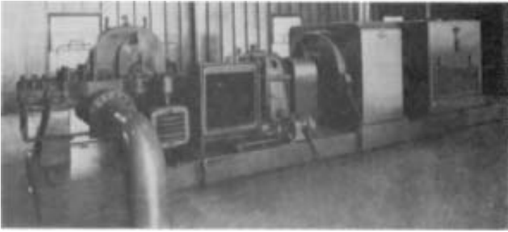
FIGURE 5 Horizontal centrifugal pump driven by a 1000-hp (746-kW), 1780-rpm induction motor through a stepup gear and an eddy-current coupling (Electric Machinery)
