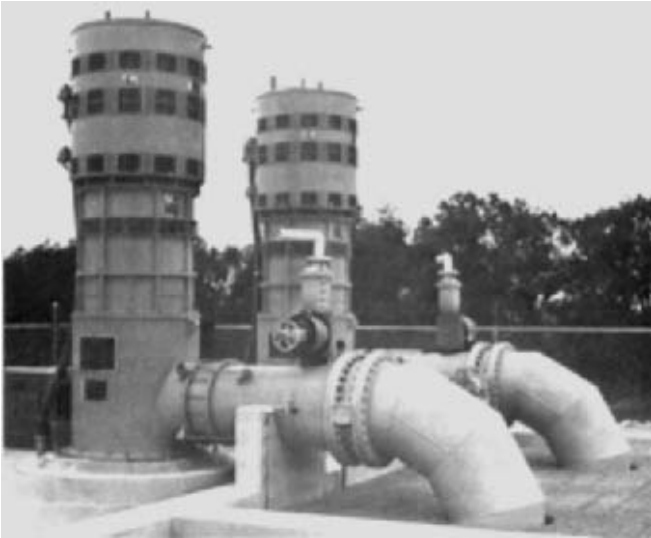
FIGURE 10 Raw water pumping station for North Texas Municipal Water District, showing vertical turbine pumps with variable-speed drives (Flowsolve Corporation)
