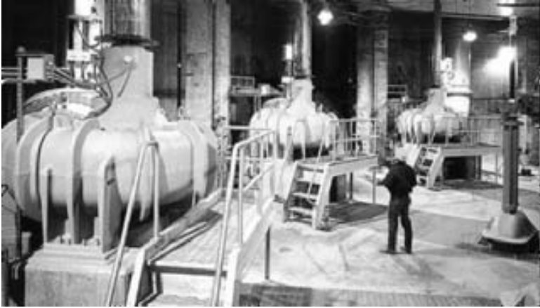
FIGURE 105 Vertical bottom-suction volute pumps installed in a sewage pumping station (Flowsolve Corporation)
