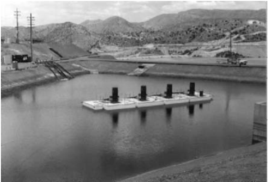
FIGURE 5 An installation of four floats with top inlet cantilevered shaft pumps (Hazleton Pumps, Inc.)
