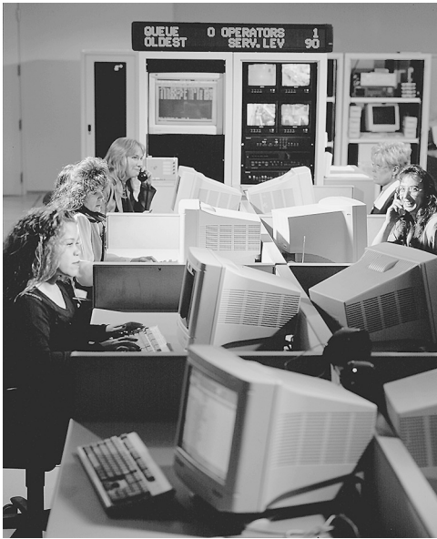
EXHIBIT 26.2 A Central Station. Notice that the display in the background indicates the signal traffic and availability to process incoming signals. (Source: SimplexGrinnell, Westminster, MA)
