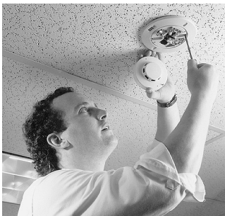
EXHIBIT 14.8 Technician Removing Wire from Device to Check Electrical Supervision. (Source: Simplex-Grinnell, Westminister, MA)
