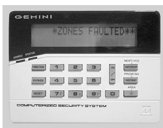
EXHIBIT 29.16 Keypad Display Arrangement. (Source: NAPCO Security Systems, Inc.—Gemini, Amityville, NY)
