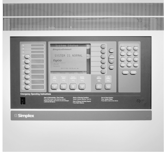
EXHIBIT 10.4 Fire Alarm Control Unit Showing Display Area and Controls for Alarm, Supervisory, and Trouble Signals. (Source: SimplexGrinnell, Westminster, MA)
