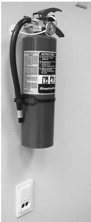
EXHIBIT 17.46 Fire Extinguisher Monitored by a Fire Extinguisher Monitoring Device. (Source: MIJA Inc., Rockland, MA)
