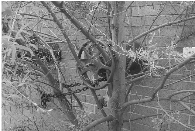
EXHIBIT 14.6 Obstructed Sprinkler Water Supply Control Valve and Supervisory Signal Device. (Source: Automatic Fire Alarm Association, Inc., Lake Mary, FL)
