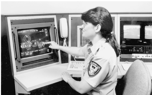
EXHIBIT 3.40 Proprietary Supervising Station. (Source: SimplexGrinnell, Westminister, MA)
