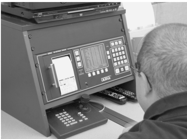
EXHIBIT 27.3 Wired Network Receiving Equipment. (Source: Lakes Region Mutual Fire Aid, Laconia, NH; photo by Debbie Kardaseski)
