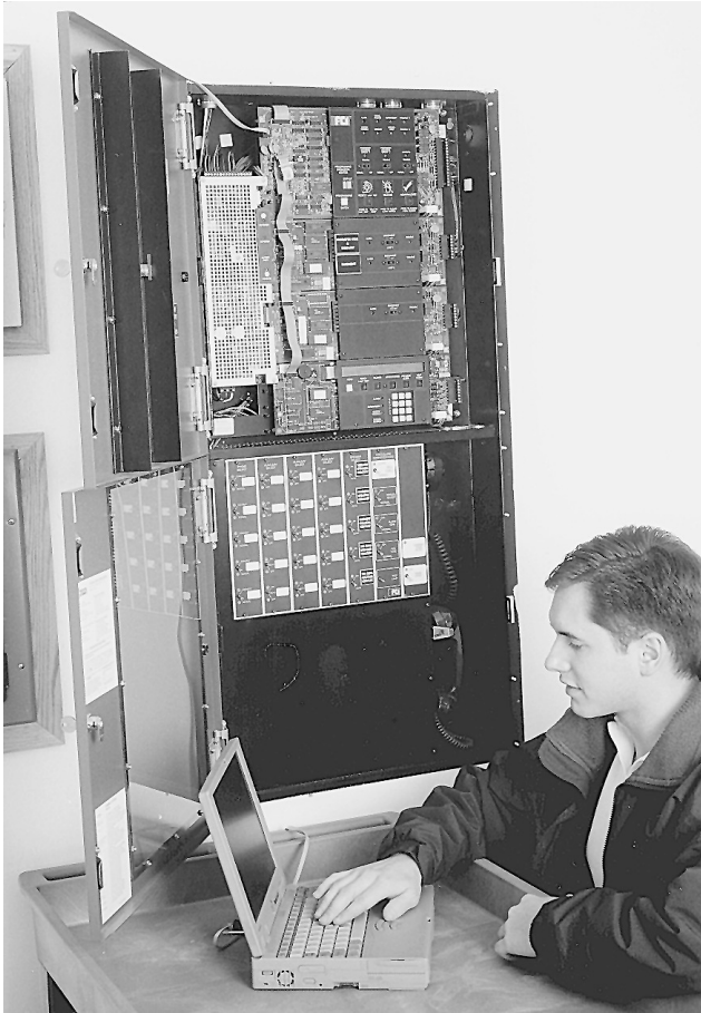
EXHIBIT 14.7 Technician Using a Laptop Computer to Modify Software. (Source: Mammoth Fire Alarms, Inc., Lowell, MA)
