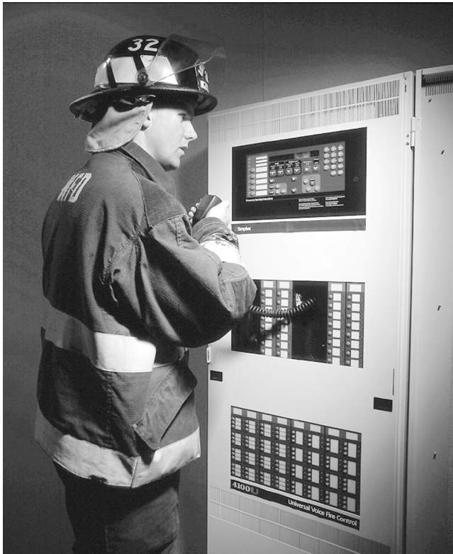
EXHIBIT 24.1 In-Building Fire Emergency Voice/Alarm Communications System. (Source: SimplexGrinnell, Westminster, MA)
