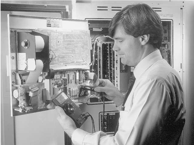
EXHIBIT 14.1 Technician Testing Fire Alarm System. (Source: SimplexGrinnell, Westminster, MA)
