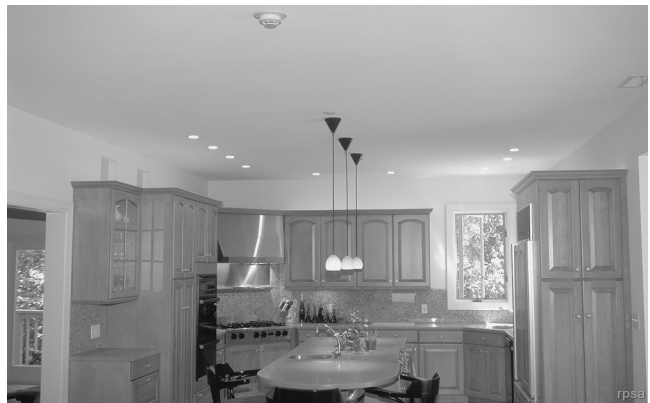
EXHIBIT 29.18 Photoelectric Smoke Detector Located Between 10 ft (3.0 m) and 20 ft (6.1 m) from a Cooking Appliance. (Source: R. P. Schifiliti Associates, Inc., Reading, MA)
