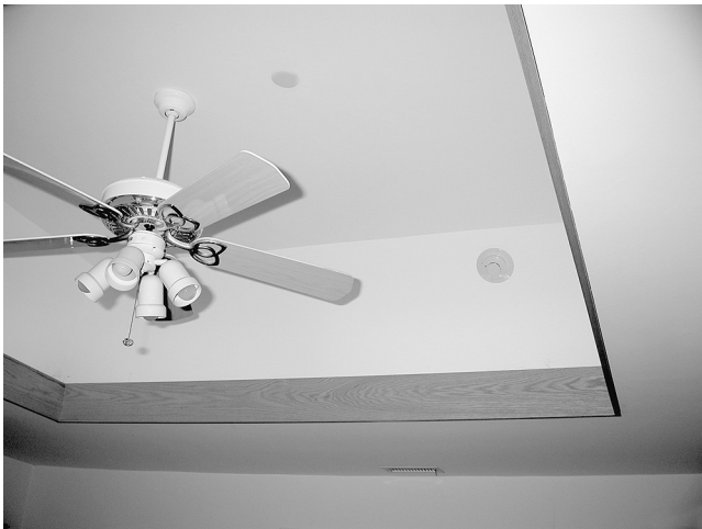
EXHIBIT 29.19 Smoke Detector Located on a Tray-Shaped Ceiling. (Source: R. P. Schifiliti Associates, Inc., Reading, MA)
