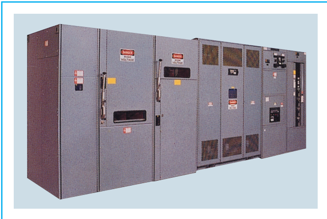
Exhibit 490.3 An assembly of metal-enclosed switchgear. (Courtesy of Square D Co.)
