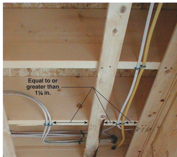
Exhibit 300.3 Nonmetallic sheathed cables adjacent to furring strips in a wood frame structure.
