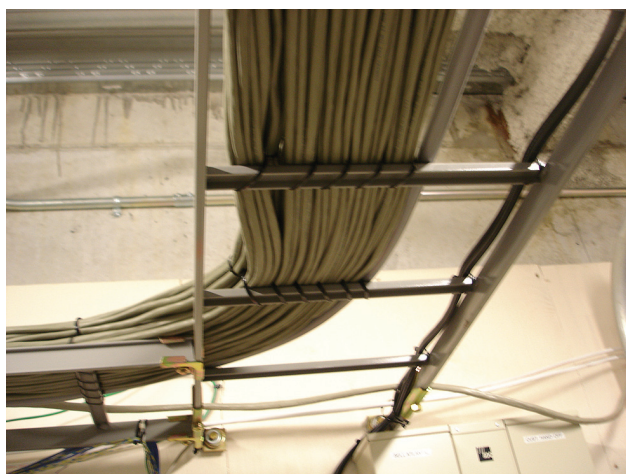
Exhibit 800.7 Overhead ladder-type cable tray containing communications cables.
