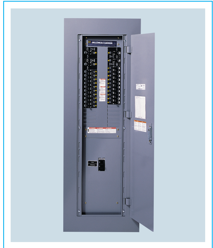
Exhibit 408.1 A panelboard with main circuit breaker disconnect, suitable for use as service equipment. (Courtesy of Square D Co.)
