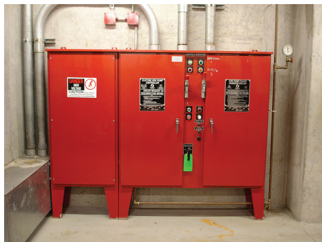
Exhibit 695.6 Listed fire pump controller and power transfer switch.
