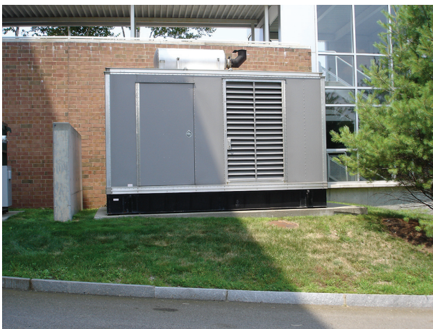
Exhibit 700.2 Alternate source of power in a heated and secure building that is located in an area not subject to flooding.
