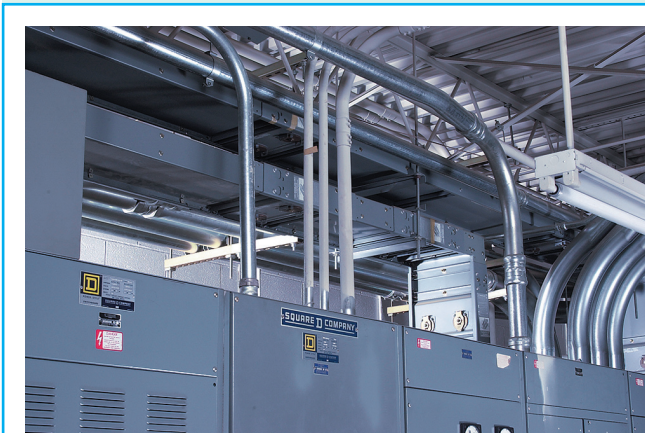
Exhibit 368.1 A 10-ft section of feeder busway.
