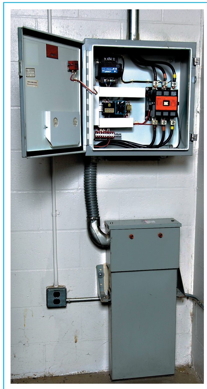
Exhibit 460.2 Power factor correction capacitors with discharge resistors.
