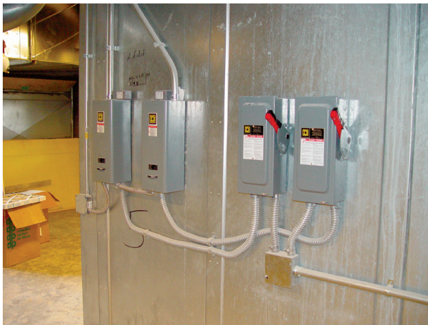
Exhibit 430.18 The disconnecting means for each controller, which must be within sight of the controller location. (Courtesy of International Association of Electrical Inspectors)
