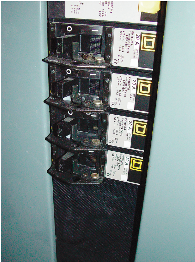
Exhibit 440.1 Four circuit breakers equipped with locking hardware that is not readily removable or transferable. (Courtesy of International Association of Electrical Inspectors)
