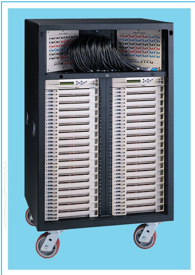
Exhibit 520.12 A large, portable SCR dimmer switchboard (rolling rack). (Courtesy of Electronic Theatre Controls, Inc.)
