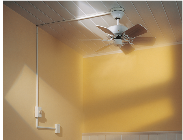
Exhibit 388.2 An example of a surface nonmetallic raceway supplying a speed control switch and a paddle fan outlet. (Courtesy of The Wiremold Co.)
