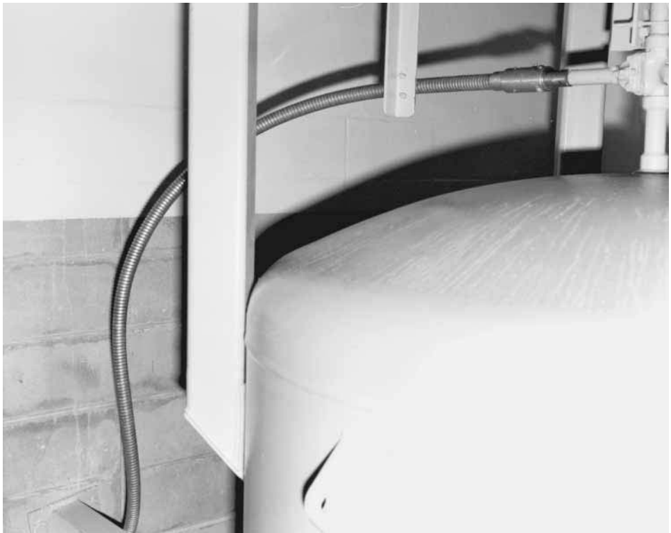
FIGURE 5.68 Flexible shaft operating valve in remote location underneath a tank.
