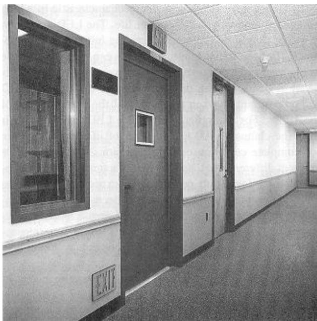
Figure 29-13. Supplemental exit signs mounted near the floor can be seen by occupants crawling along the floor in smoky conditions.
