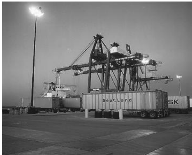
Figure 19-33. High-mast floodlights located to illuminate the dock area while reducing glare for the crane operators and cargo handlers.
