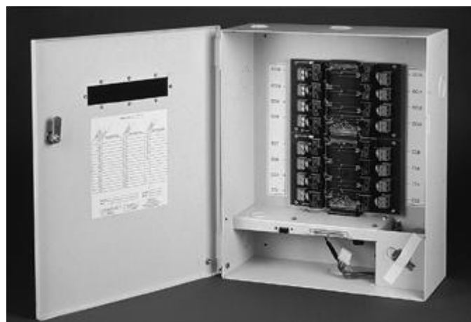
Figure 26-6. An example of a central lighting control system based on programmable time-of-day operation of relays and low-voltage switching.
