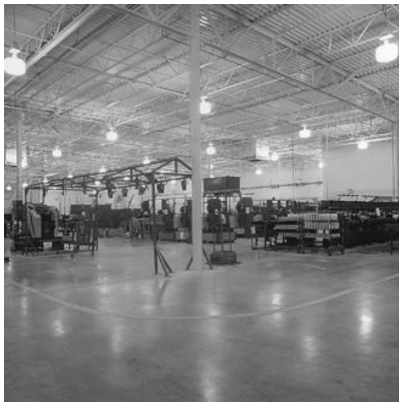
Figure 19-11. Semidirect HID luminaires mounted from the roof structure. Uplight improves the visual environment. The bottom of the luminaires is usually located above the bottom chord of the lowest truss.
