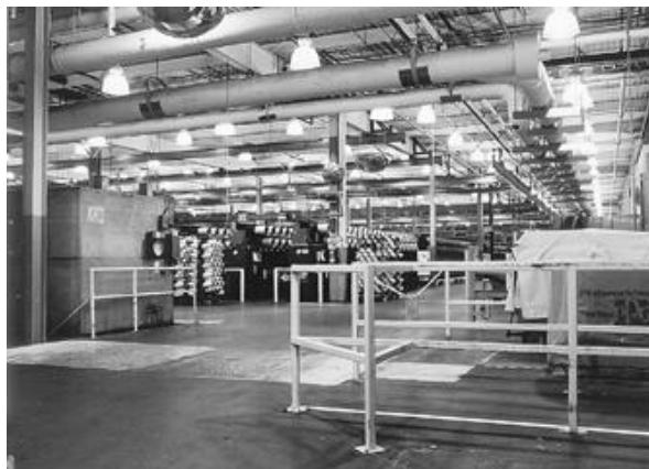
Figure 19-19. Lamp selection should include consideration of color rendering safety indicators such as exit signs and floor stripping.
