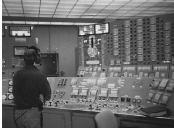
Figure 19-28. Control room of a nuclear generating station with a louvered ceiling.
