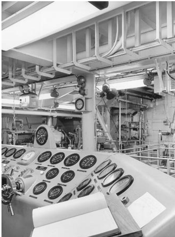
Figure 23-27. Lighting for the engineering control console is provided by fluorescent luminaires. Care should be taken to avoid glare and veiling reflections.
