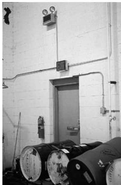
Figure 29-4. This wall-mounted sealed-beam unit provides emergency lighting for fire-fighting equipment (the fire extinguisher) as well as the exit approach that should be kept clear of obstructions (e.g., the barrels shown here).
