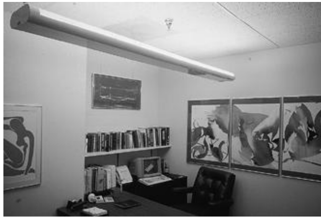
Figure 11-9. Pendant luminaires are commonly used to provide indirect illumination.
