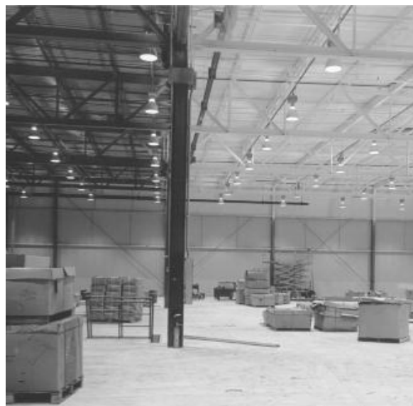
Figure 19-8. The importance of a white ceiling in an industrial facility is shown in this plant under construction. Note the improved visual environment in the right bay (where the painters have finished the ceiling) compared to that in the left (as yet, unpainted). The illuminance in the right is substantially higher, too.
