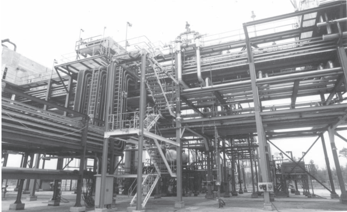
Fig. 19.2 Piperack/cablerack junction with valve access station – requires forethought and planning
