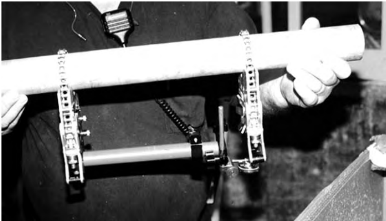
FIGURE 6.58 Observe the amount of sag on the dial indicator as you rotate the assembly to the six o'clock position.
