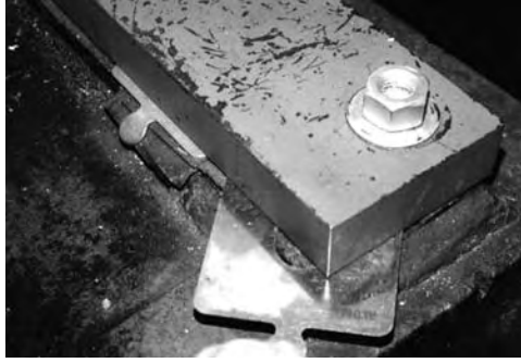
FIGURE 3.69 Inspection of the grout under the soleplate revealed that the grout had begun to deteriorate. Apparently this was observed prior to this and precut shim stock was used to attempt to correct the gap between the top of the grout and the underside of the soleplate, which is not recommended. Also notice that the top of the anchor bolt is not fully engaged in the nut.
