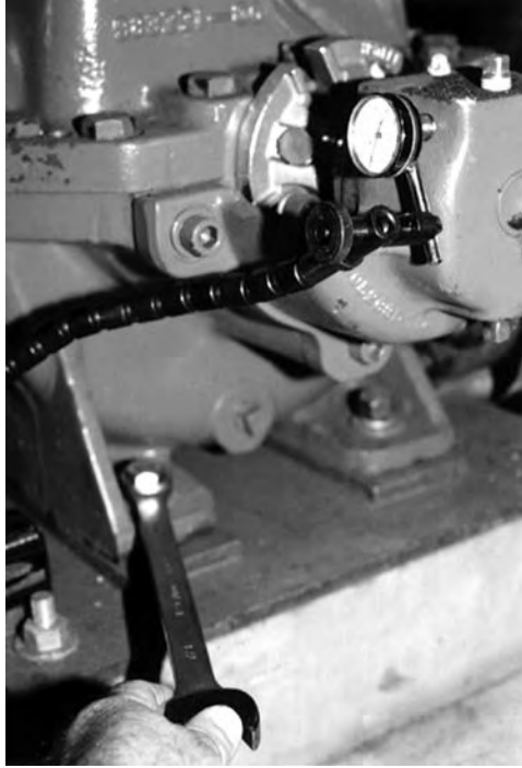
FIGURE 3.74 Alternate piping stress check using magnetic base and indicator to observe case movement when foot bolts are loosened with piping attached.
