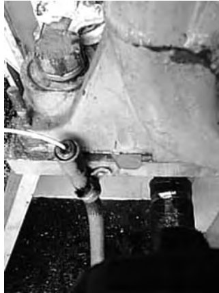
FIGURE 5.51 Soft foot correction shims for a pillow block bearing on a fan.
