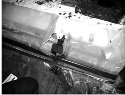
FIGURE 3.50 Grout leak around form.
