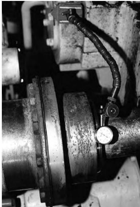
FIGURE 5.24 Measuring runout on the backside of the gear coupling hub attached to a steam turbine.
