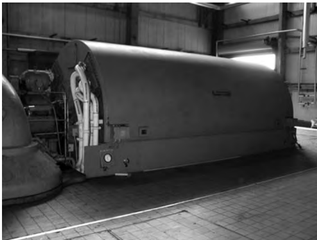
FIGURE 21.57 Typical alternating current electric generator.
