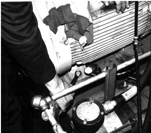
FIGURE 5.52 Checking for lift with a magnetic base and dial indicator on a machine foot.
