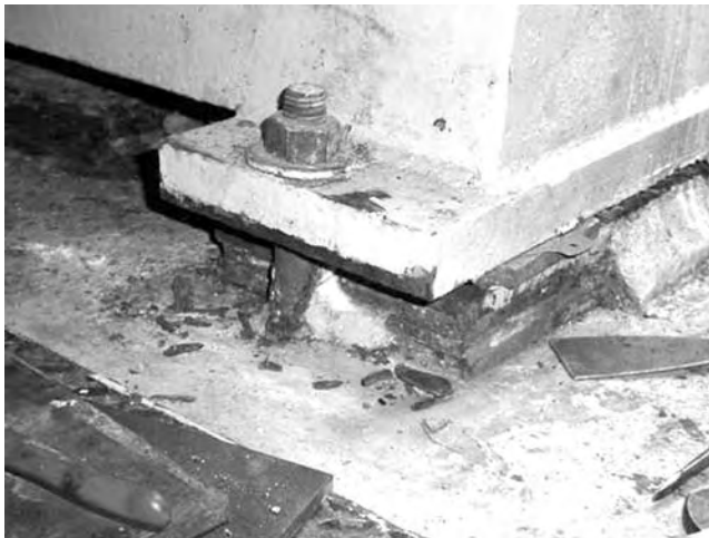
FIGURE 21.81 Corner of gearbox in Figure 21.80 showing that the foot bolt is not supported on the outer edge (in addition to the soft foot problem shown in Figure 21.83).
