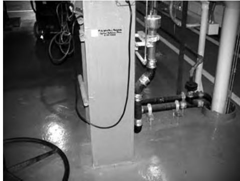
FIGURE 3.61 Reference target on building column used to buck in to same elevation.
