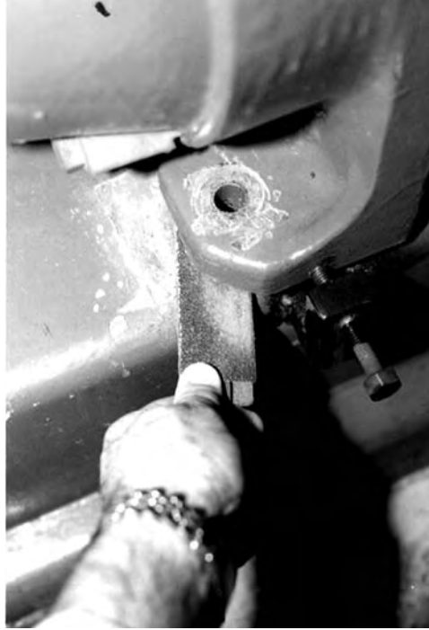
FIGURE 5.46 Cleaning the pump feet using 180 grit emery cloth wrapped around a 1/8 in. thick steel bar and “sawing” back and forth to clean the underside of the machine foot and the base plate at the same time.
