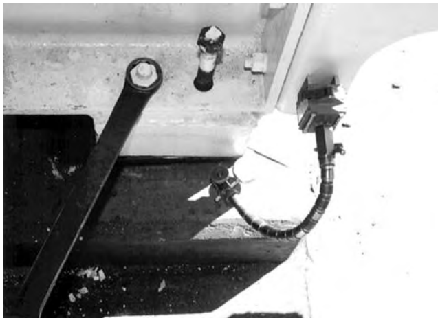
FIGURE 5.58 Checking for lift after installing the noncontact (i.e., soft foot) correction shims.
