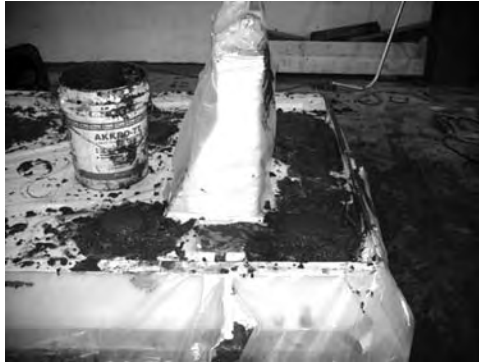
FIGURE 3.53 Grout began swelling at low end.
