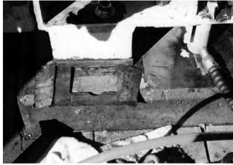
FIGURE 5.37 Machine frame to sole plate shim pack that had worked loose due to a soft foot condition.
