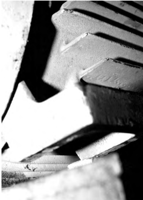
FIGURE 5.47 The underside of this motor foot is “hollow.” Make sure for using the right size shims to get as much contact as possible here.
