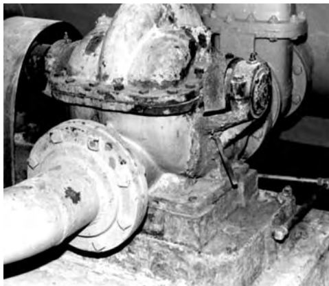
FIGURE 3.70 A misalignment condition between the motor and water pump caused the packing to leak. Over time, the spraying water severely oxidized the pump casing and baseplate.
