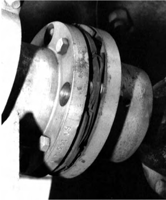
FIGURE 1.1 Disk coupling failure due to shaft misalignment.
