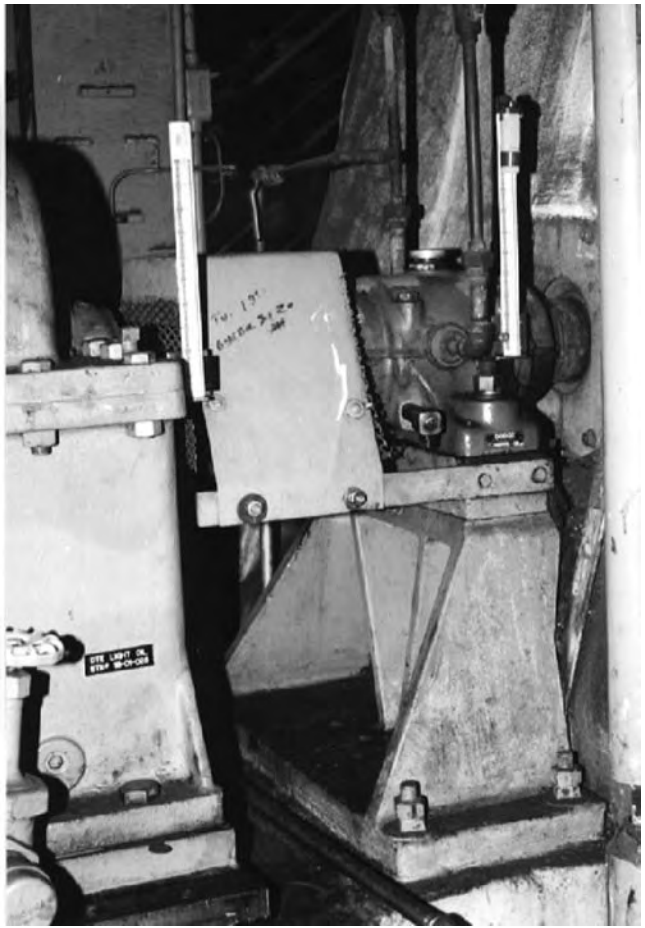
FIGURE 16.38 Scale targets mounted on gearbox and fan bearing near their centerline of rotation.
