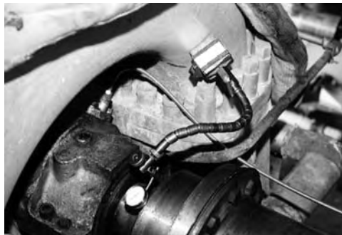
FIGURE 5.25 Measuring runout on the backside of a gear coupling hub attached to a compressor.
