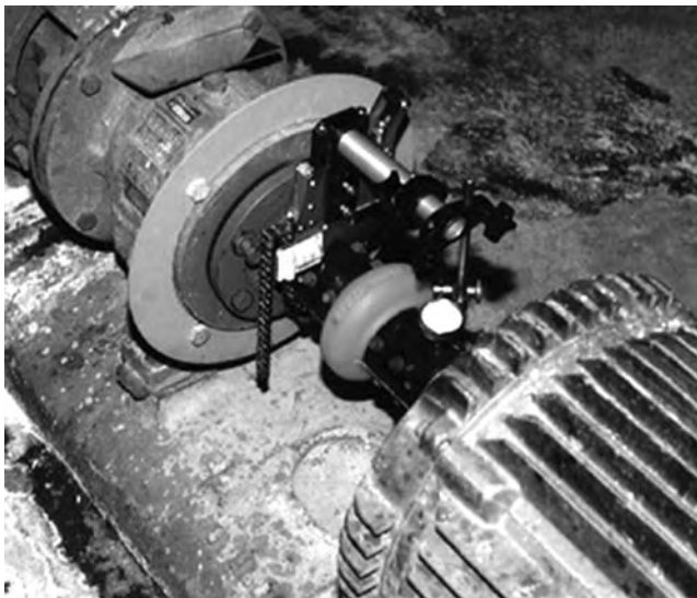
FIGURE 6.35 Dial indicator positioned at twelve o'clock and zeroed.
