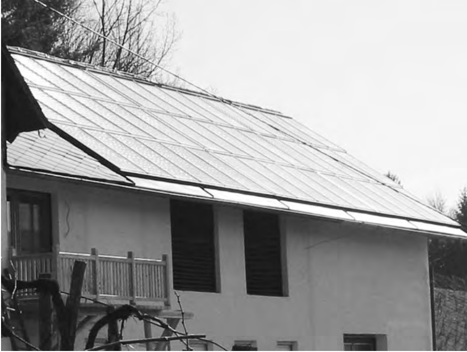
FIGURE 20.39 Wine cooling and bottle washing, Austria. Installed capacity: 70 kW th . (From S.O.L.I.D. GmbH, Austria. With permission.)
