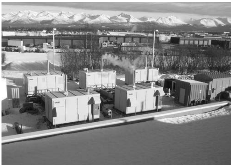
Fig. 20.11 Photograph of five PC25 fuel cell units installed at Anchorage, Alaska. (Courtesy of International Fuel Cells Inc.)
