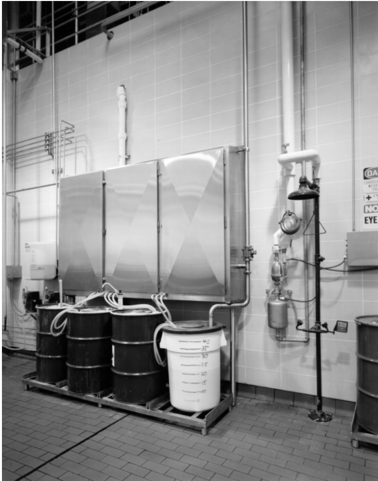
FIGURE 15.4 Chemical pump enclosure — supply containers and safety shower in a dairy processing facility.
