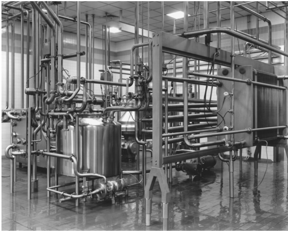
FIGURE 15.20 This HTST is equipped with a CIP constant level tank supplied through a U-bend transfer panel.
