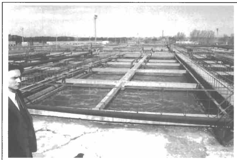
Figure 45. Rectangular settling basins in operation.
