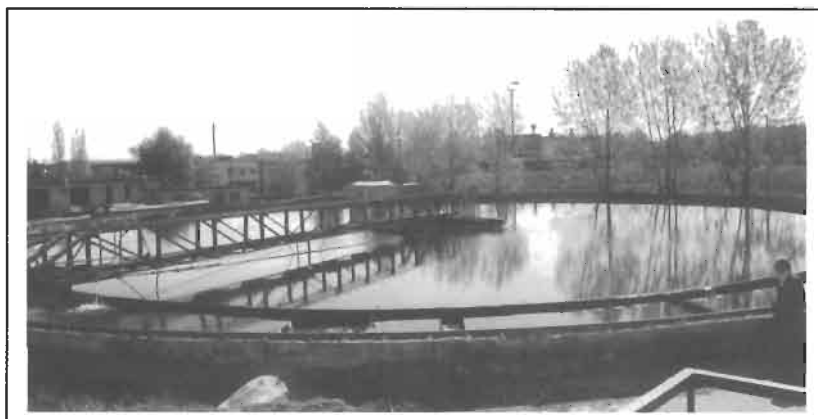
Figure 44. Clarifier in operation in a wastewater treatment plant at the Avtovaz auto-making plant in Russia.
