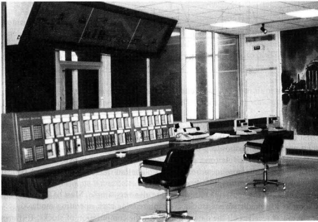
Fig. 46.15. Control room of a pan station (the two management computers are on the right).
