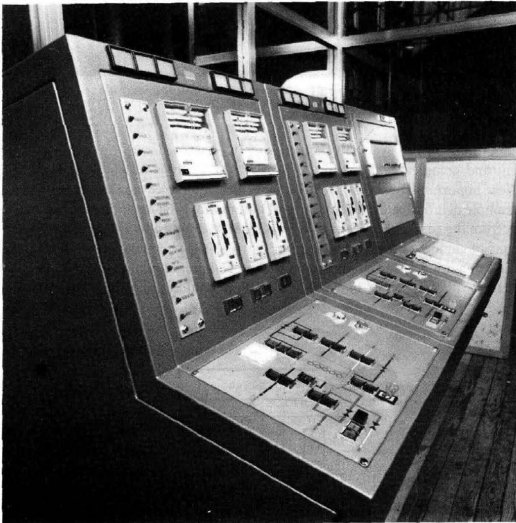
Fig. 46.3a Control cabinet for vacuum pan.
