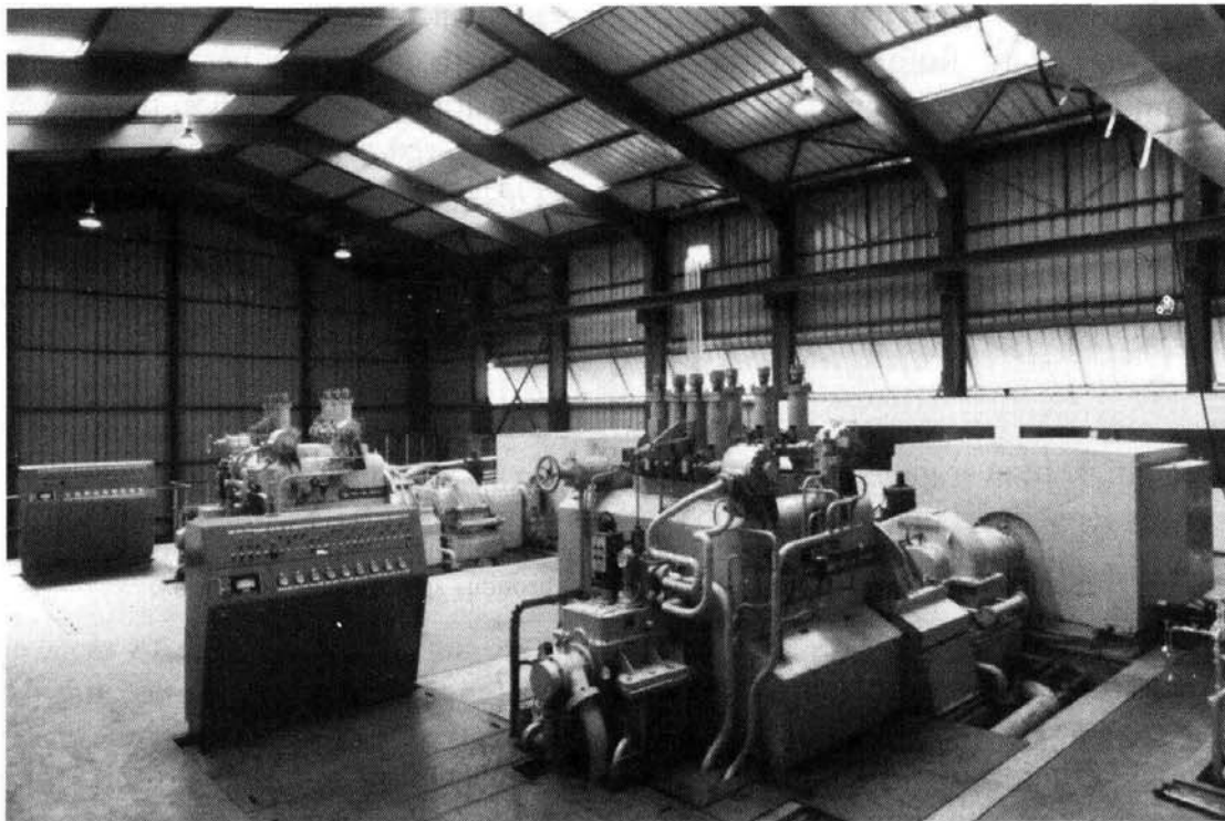
Fig. 43.20. Group of two condensing turbo-generators (40 bar - 400°C. Extraction at 1.5 bar).
