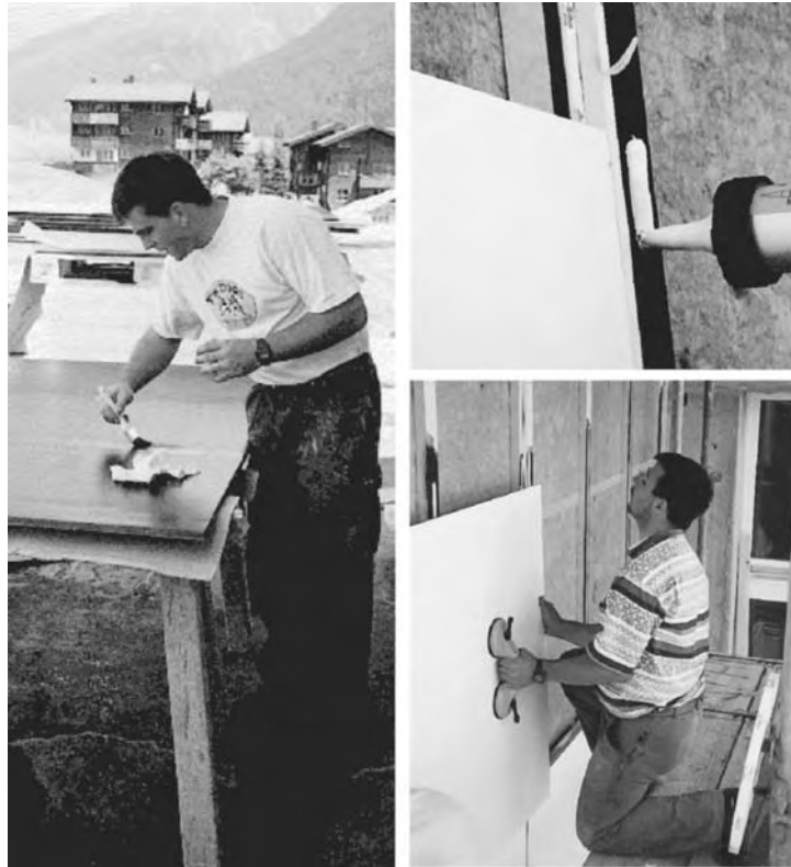
Figure 106: Priming of the contact surface (left), gunning of triangular bead of adhesive (top right), positioning of the panel (bottom right).
