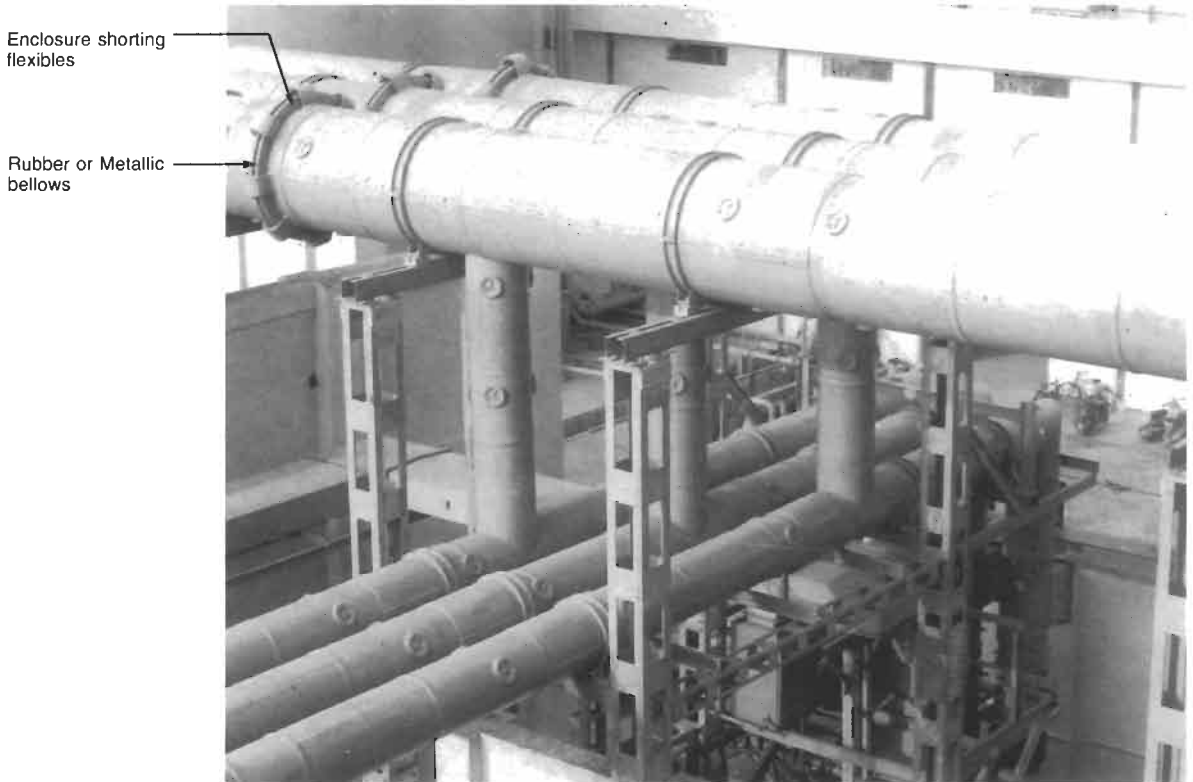
Figure 31.4(c) 24 kV, 20 kA, IPB straight run and tap-offs (Courtesy: Controls and Switchgears)
