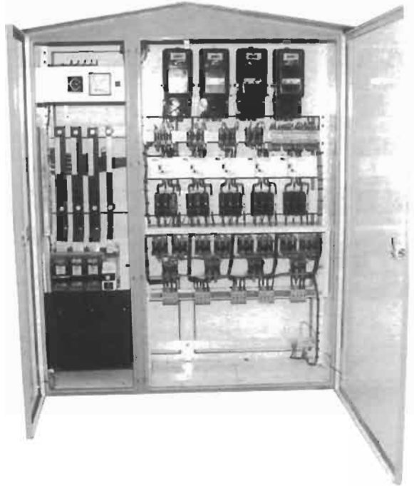
Figure 13.4 A non-compartmentalized distribution board
