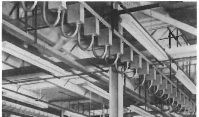
Installation of overhead bus system with tap-off boxes in a large assembly shop
