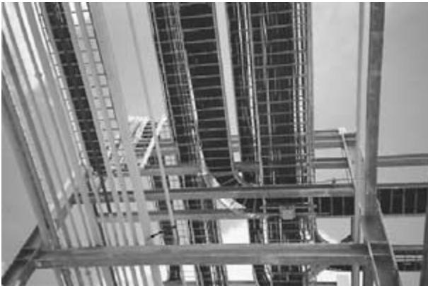
Cables of different systems are installed into different cable trays.
