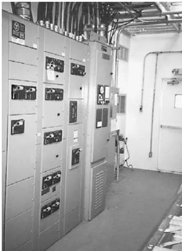
Motor control center.
