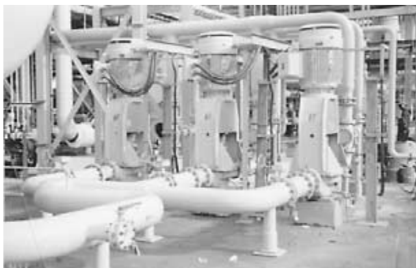
Induction motors driving pumps in industrial facility.
