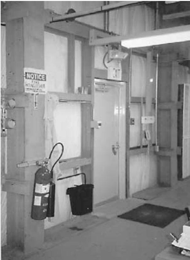
Illumination for egress paths must be provided in manned installations.
