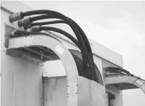
Medium-voltage cables leaving cable tray and entering switchgear building.
