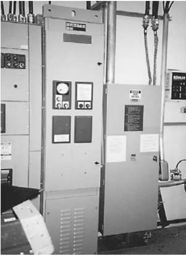
Switchboard and transfer switches require working clearance in front, but not to the side.
