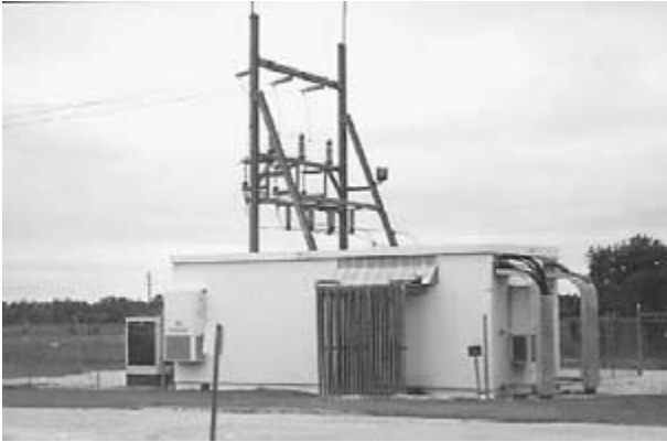
Industrial plants commonly incorporate prefabricated switchgear buildings.
