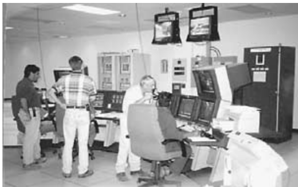
Control room of an industrial facility.
