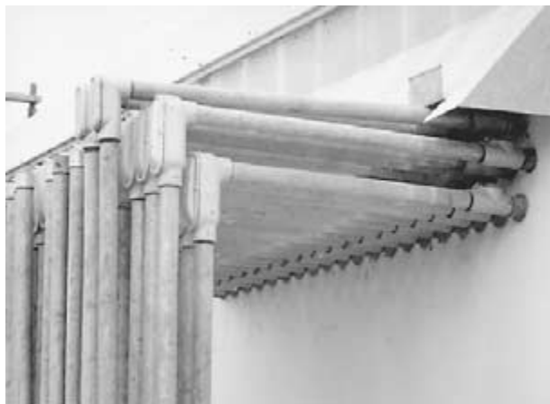
Heavy-wall rigid steel conduit in an industrial plant.
