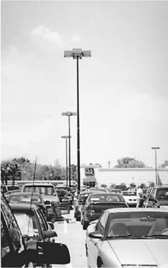
Parking lot lighting using HID lamps.
