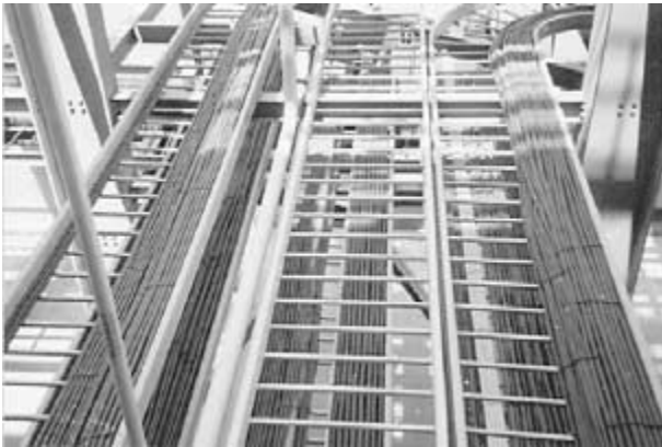
Cables in ladder cable tray.
