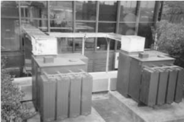
Service conductors to commercial building in the form of bus duct.
