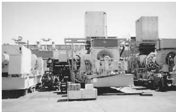
Gas-turbine generators arrive at the installation site prepackaged on skids.
