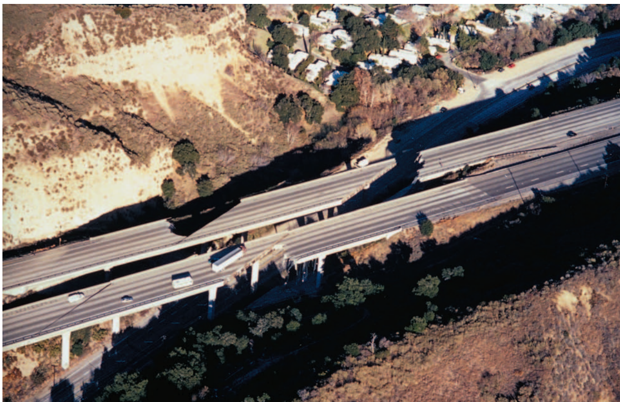
Aerial view of Interstate 5, a California highway damaged by the Northridge earthquake in January 1994. Photograph by Robert A. Eplett. Governor's Office of Emergency Services.
