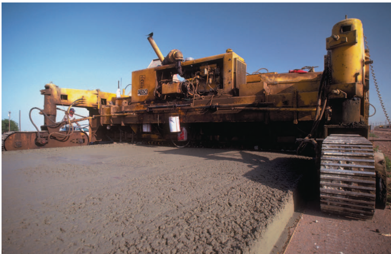
Concrete being used to pave a road. Photograph by Chris Jones. Stock Market. Reproduced by permission.
