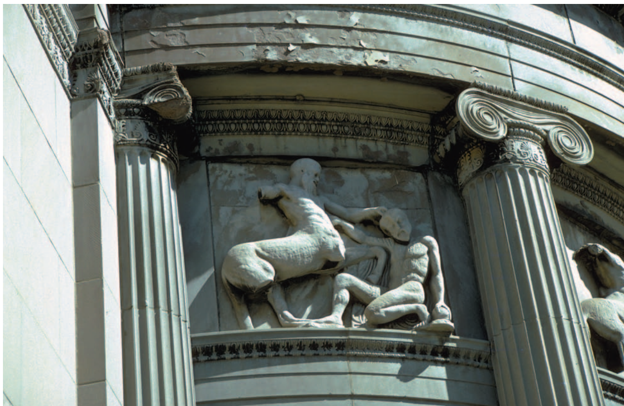
Acid rain damage done to a piece of architecture in Chicago, Illinois. Photograph by Richard P. Jacobs. JLM Visuals. Reproduced by permission.
