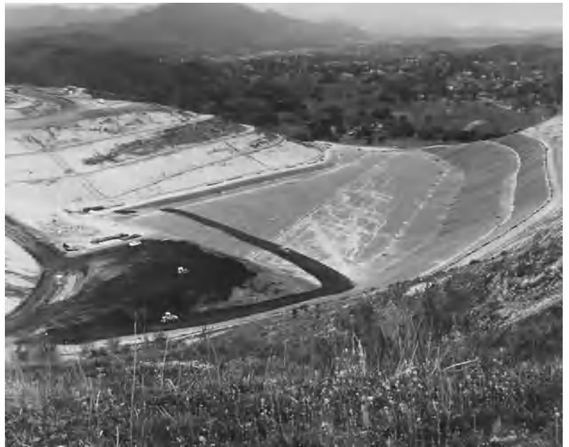
Fig. 4. Calabasas solid-waste landfill in Los Angeles County, California, being lined with geomembrane.
