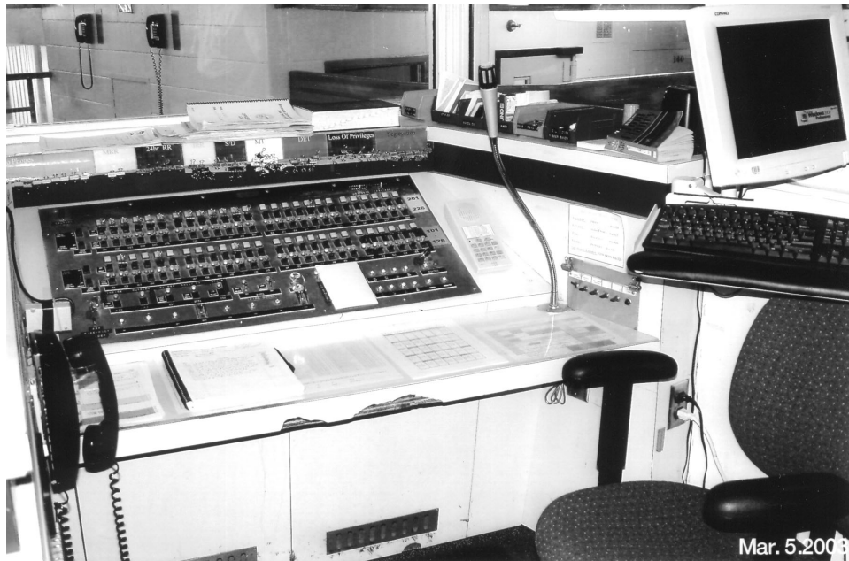
Photo 2 View of the control station
