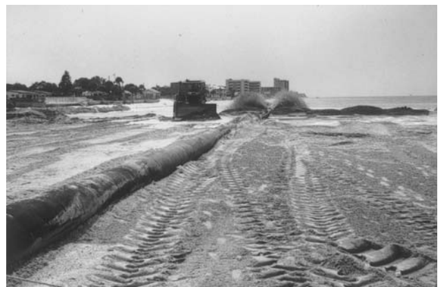
Figure H17 Pumping and spreading nourishment sand in the construction of a new beach.
