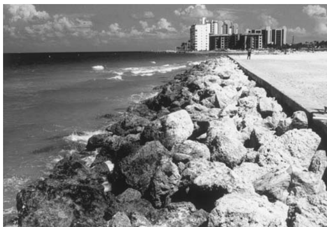
Figure H11 Rip-rap in front of concrete seawall. This is one of the most common types of erosion protection on the open coast environment.
