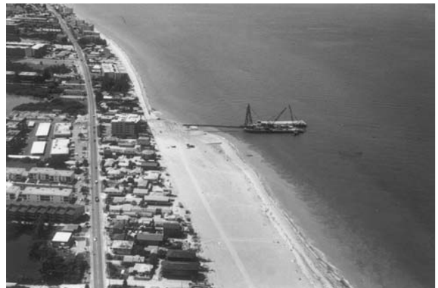
Figure H16 Construction of a new beach using a conveyor belt to offload sand from a large barge.
