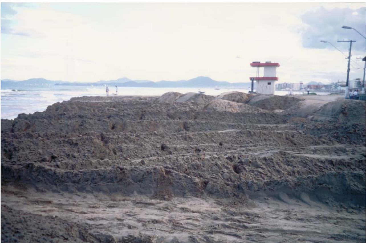
Figure B29 Emergency beach renourishment at Gravatá Beach, Santa Catarina, Brazil. A coastal highway and commercial infrastructure was threatened by beach erosion during a strong southeaster that brought heavy surf conditions to the coast during the Southern Hemisphere winter of 1999. Removal of the beach by wave and current action, undermined part of the coastal highway interrupting coastal access. Although of finer grain size than the native beach sand, emergency fill was trucked to the site for immediate shore protection.
