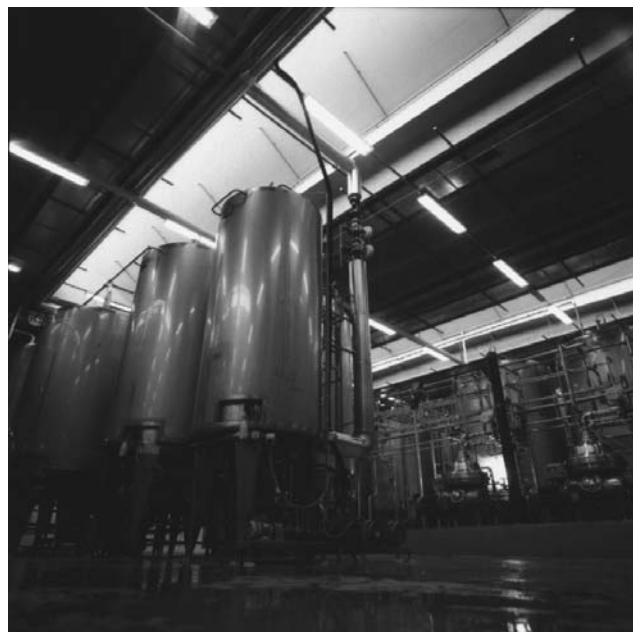
Figure 2. Insulin production plant.
