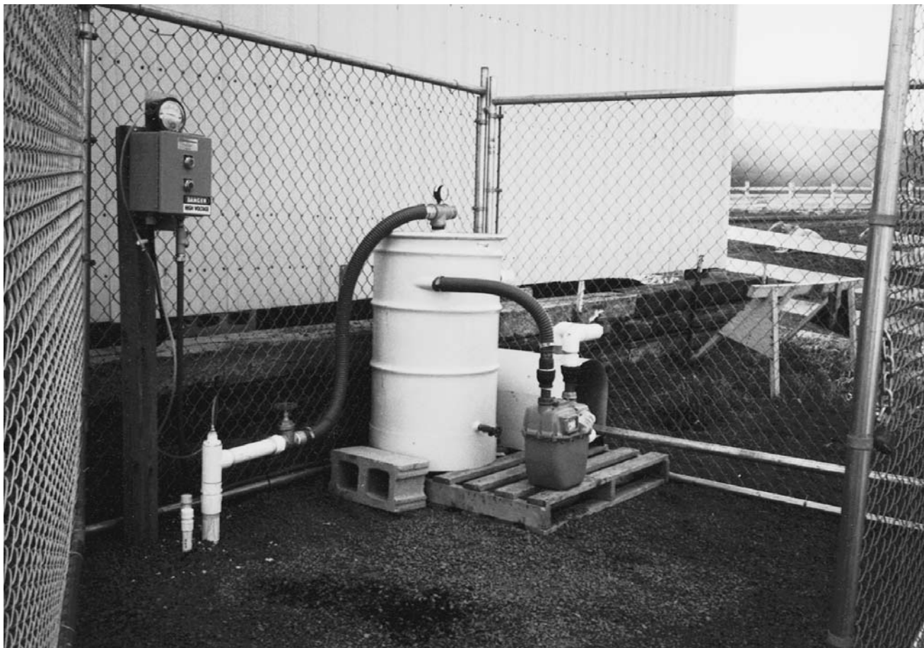
Figure 2. Petroleum bioventing operation. Source: University of Idaho, with permission.
