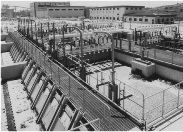
Figure 9. Photograph of denitrification plant using charged photo-cross-linked resin gels in Tokyo. Nitrifying tank volume, 10,000 m 3 , Packing ratio of gel, 10%.
