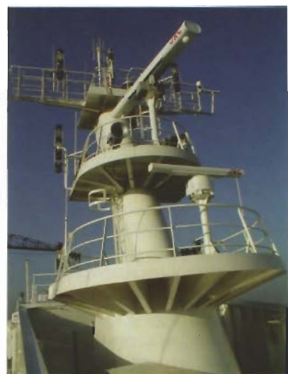
Top deck of a modern ship showing the compromise in installation of a transmitting disturbing radar aerial and the VHF receiver aeriels.
