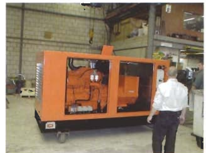
An emergency generator
