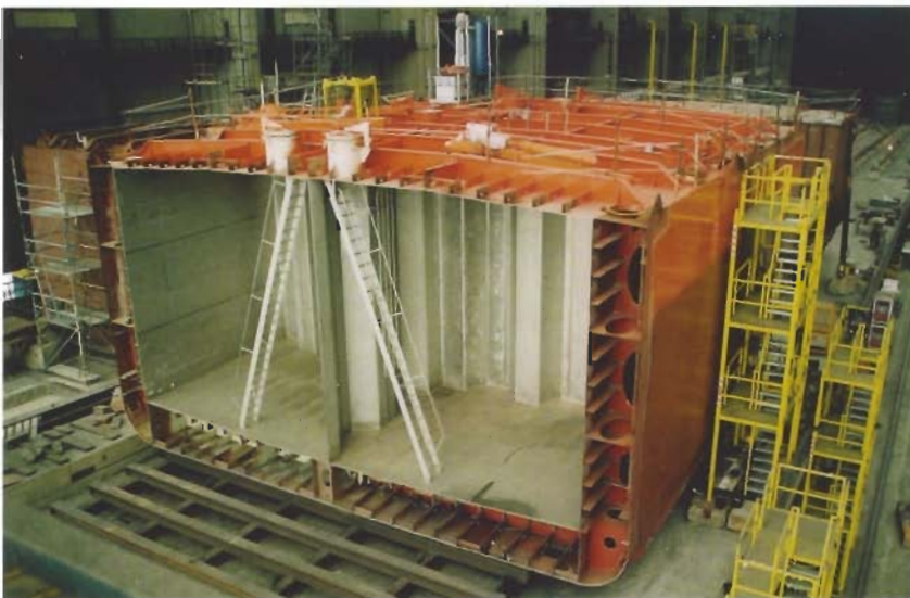
Another view of the same tank
