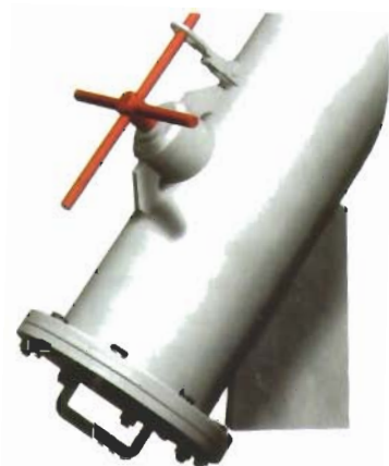
Pipe outside the chain locker, where the end link is connected. The wheel is used to secure a pin through the end link.
