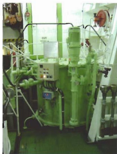
Bilge water separator with 15 ppm oil content meter / alarm
