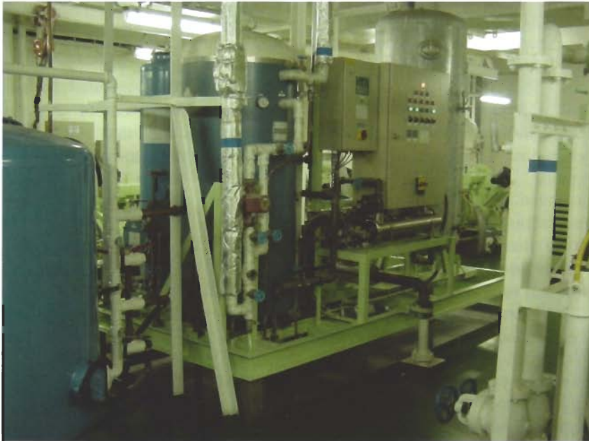
reverse osmosis plant
