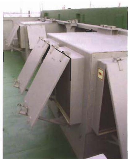
Ventilation grill with cover
