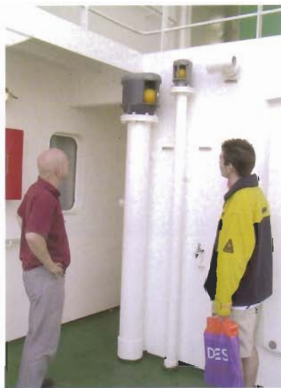
Raised tank vents
