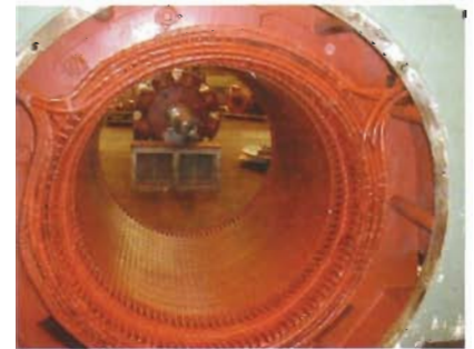
AC generator under maintenance
