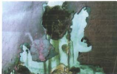
Seven years of damage to the paintlayer. The cause: badly protected welded seams which may be caused by insufficient cleaning after welding prior to painting.
