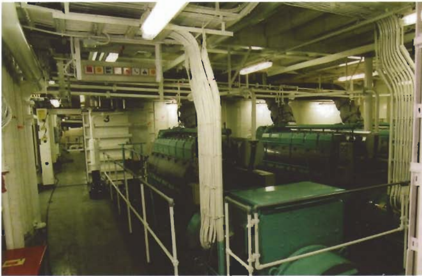
Auxiliary engine room of a ferry
