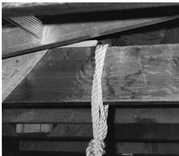
Figure 1 Photograph showing multiple grooves worn into the beam with rope in situ. Demonstrates evidence of prior autoerotic activity of a similar nature.
