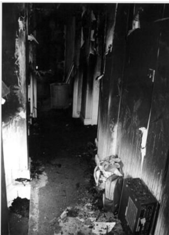
Figure 3 Typical smoke-logging in a passageway. Hot, buoyant smoke produces staining at a high level.
