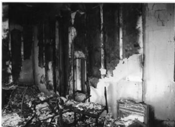
Figure 2 A characteristic funnel pattern indicating an armchair as the point of ignition. The fire had, in fact, been ignited approximately 500 mm from the chair, but had spread to it at an early stage in the fire.
