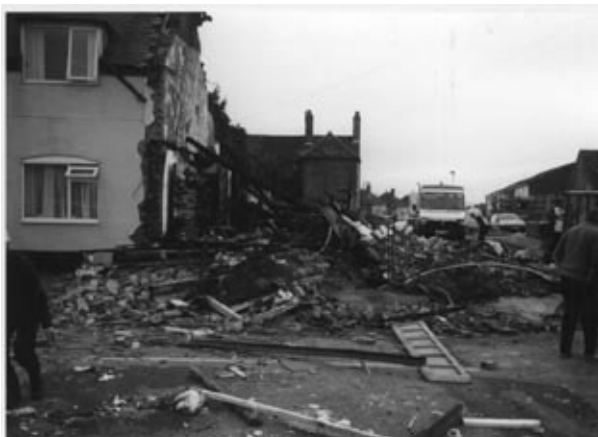
Figure 5 A typical petrol vapor explosion, which caused almost complete demolition of the building, followed by a widespread and destructive fire.
