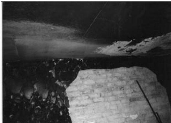
Figure 1 Plaster spalled from a wall as a result of cooling by fire fighting jets. The direction of the spray can be seen from displaced soot on the ceiling.
