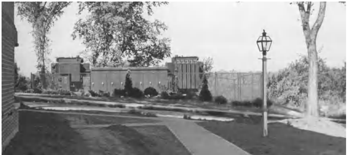
Fig. 2. View of a residential outdoor distribution substation with double-ended underground supply to transformers which are positioned at either end of the metal-clad switchgear.
