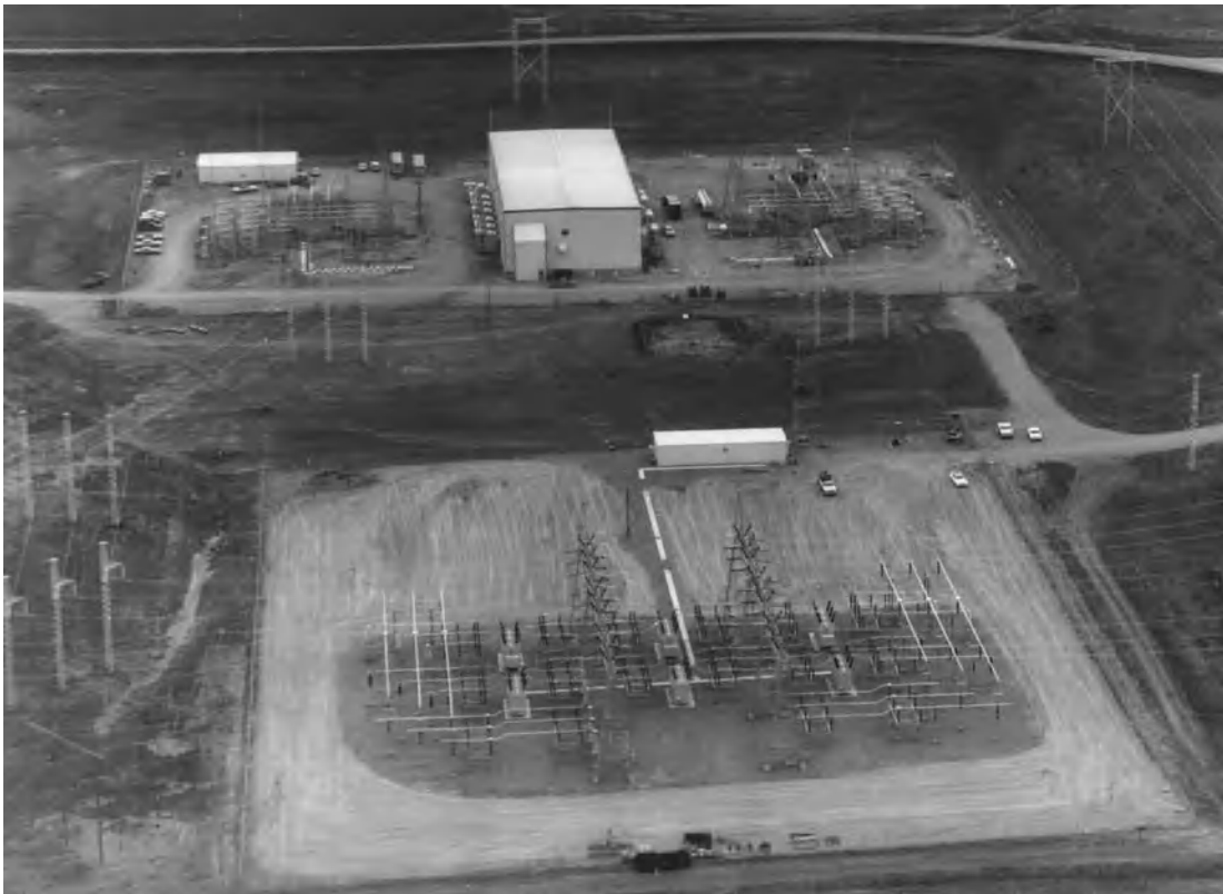
Fig. 3. View of \pm 250 -kV 500-MW HVDC converter station (upper part) and 245-kV ac substation (lower part). The large building of the converter station contains all the thyristor valves. (General Electric Co.)
