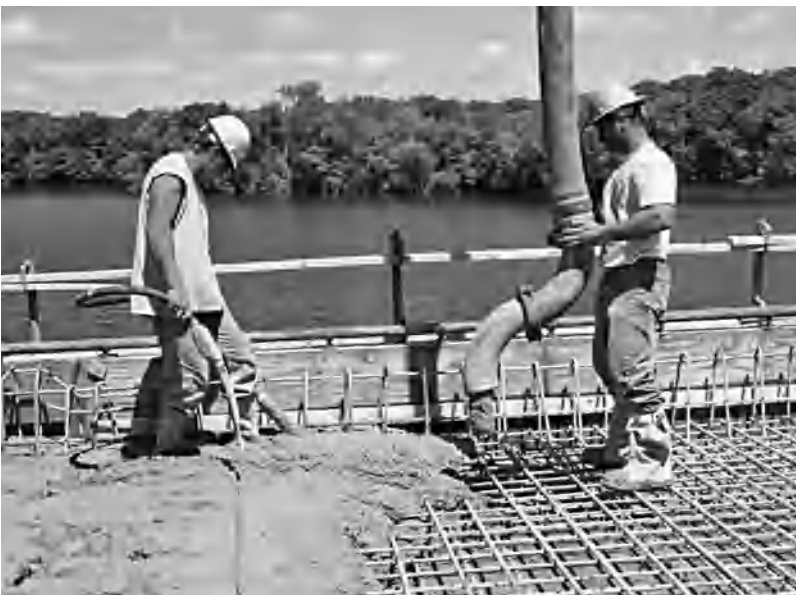
Fig. 1. Workers placing and vibrating concrete on a bridge deck including epoxy-coated reinforcing steel. (Portland Cement Association)
