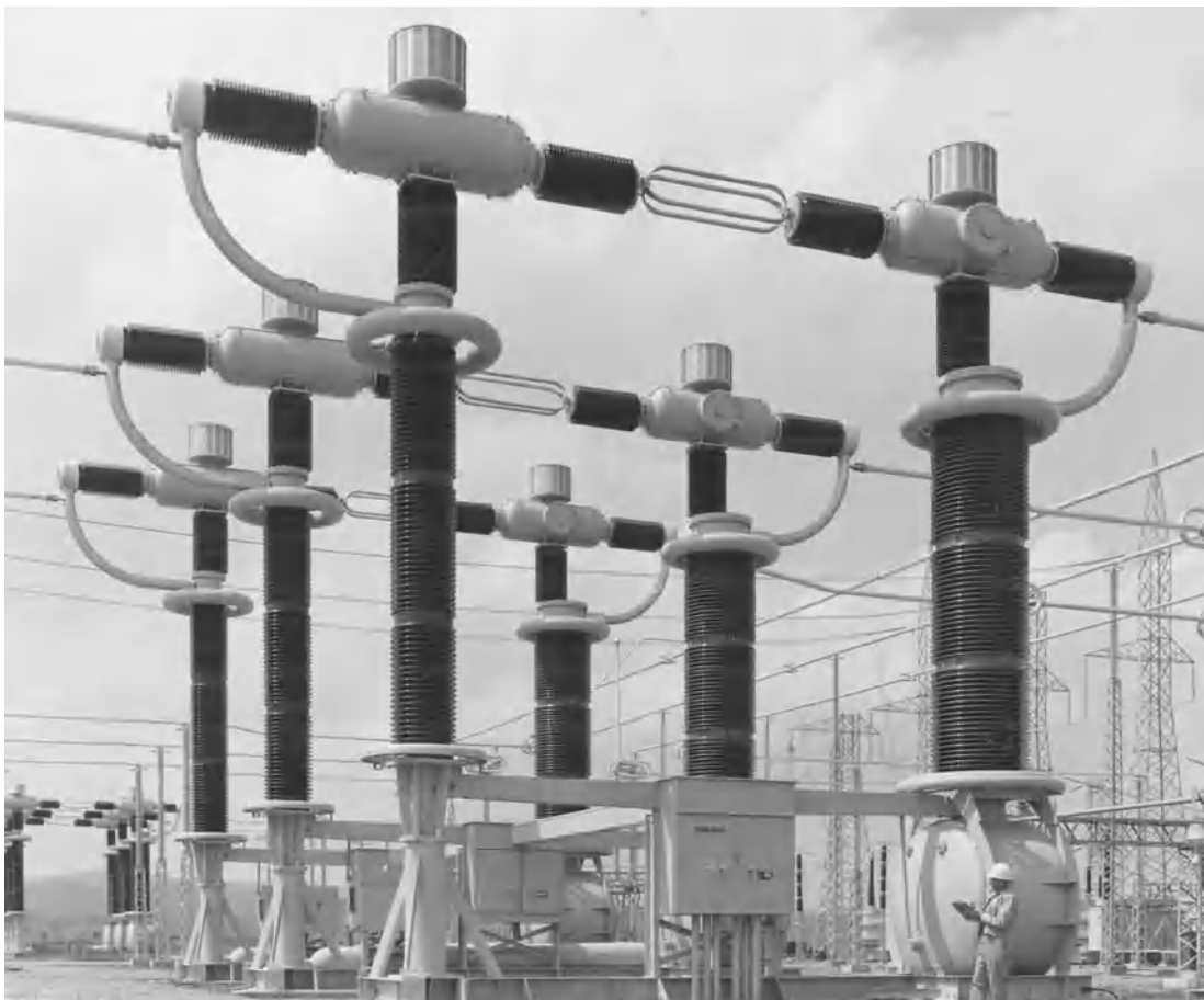
Fig. 3. Air blast circuit breaker rated for 500 kV.
