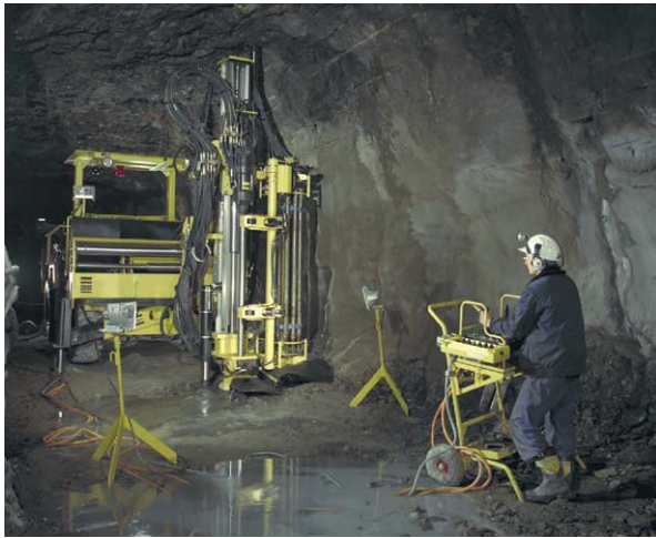
Figure 3 Underground exploration drilling (Simba H1354 for Echo Bay, Canada). Photograph by Atlas Copco.
