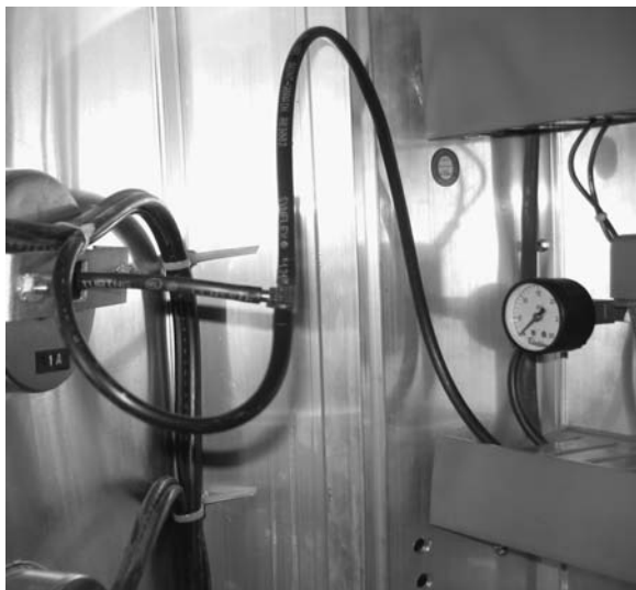
Fig. 5 Use of T-fitting to pick off fan discharge temperature signal to control fan coil valves.
