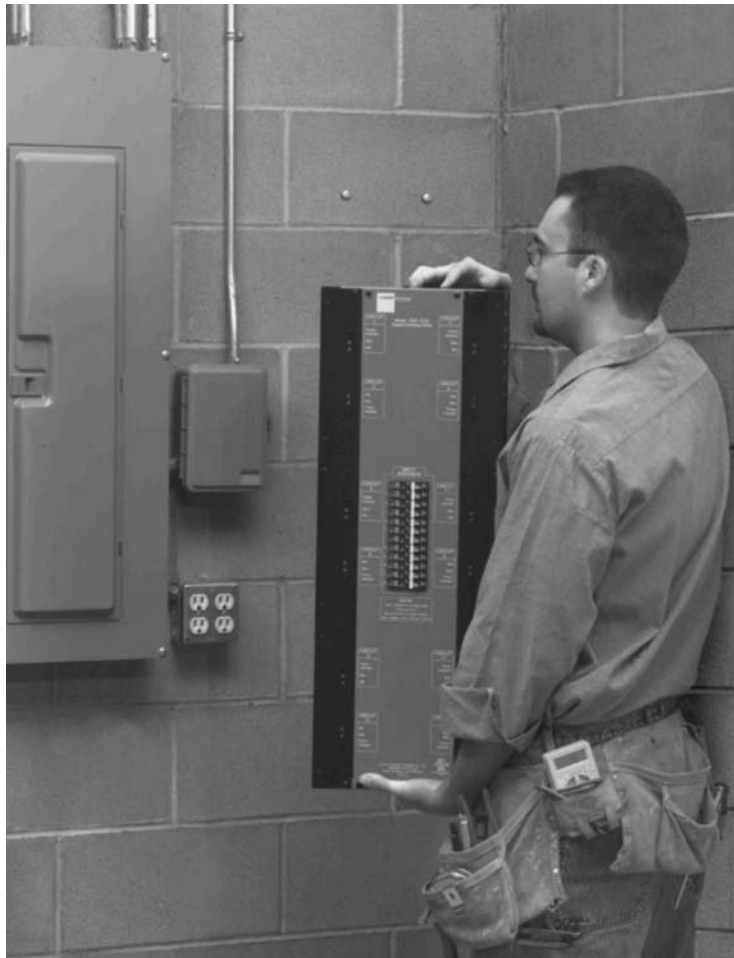
Fig. 4 Lighting control panel installation. Source: From HUNT Dimming.
