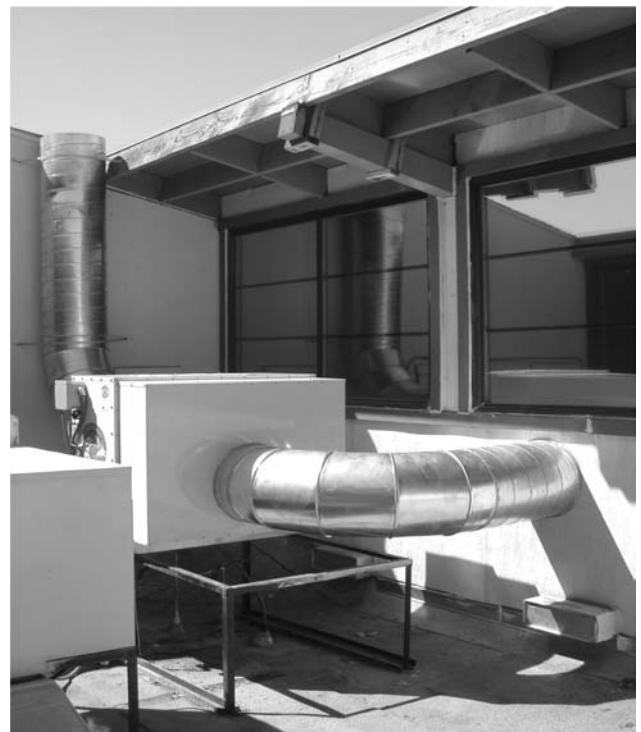
Fig. 18 Coolerado Cooler installation at a school in Sacramento, California. Source: From Sacramento Municipal Utility District (see Ref. 7).
