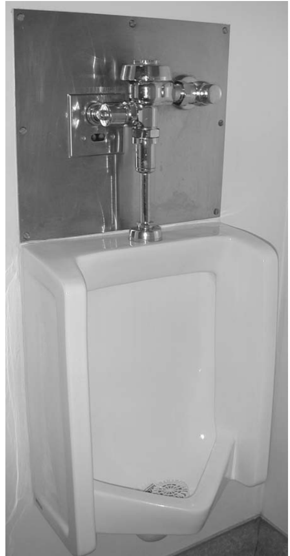
Fig. 5 Urinal with infrared sensor.
