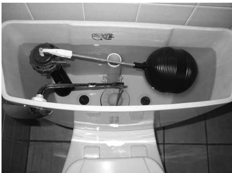
Fig. 3 Inside of tank toilet.
