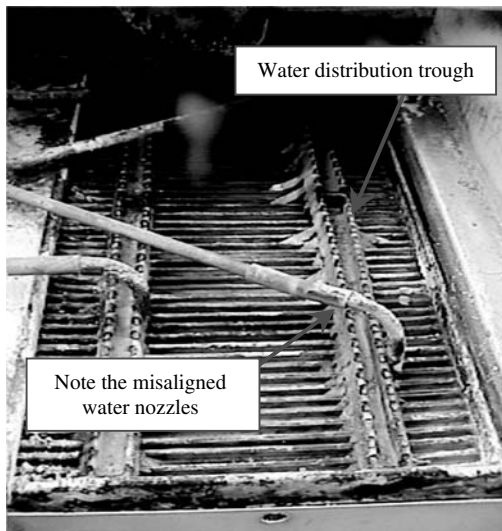
Fig. 10 The heat exchanger of this IDEC was rendered useless by misaligned water nozzles. Note also the presence of hard-water scale. This system was not equipped with a bleed line. Source: From Sacramento Municipal Utility District (see Ref. 7).
