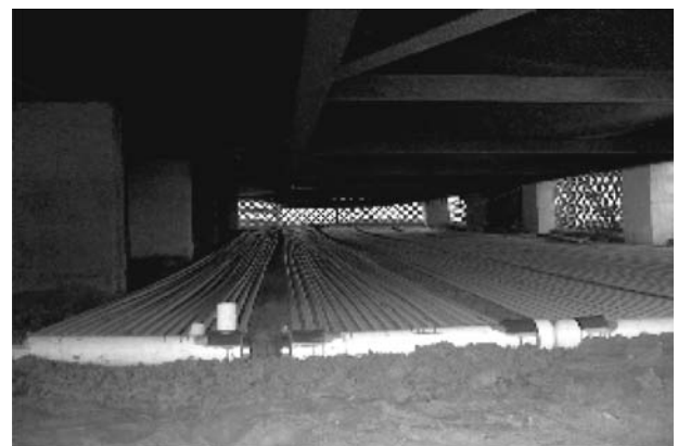
Fig. 3 PVC heat exchangers installed at DDES.
