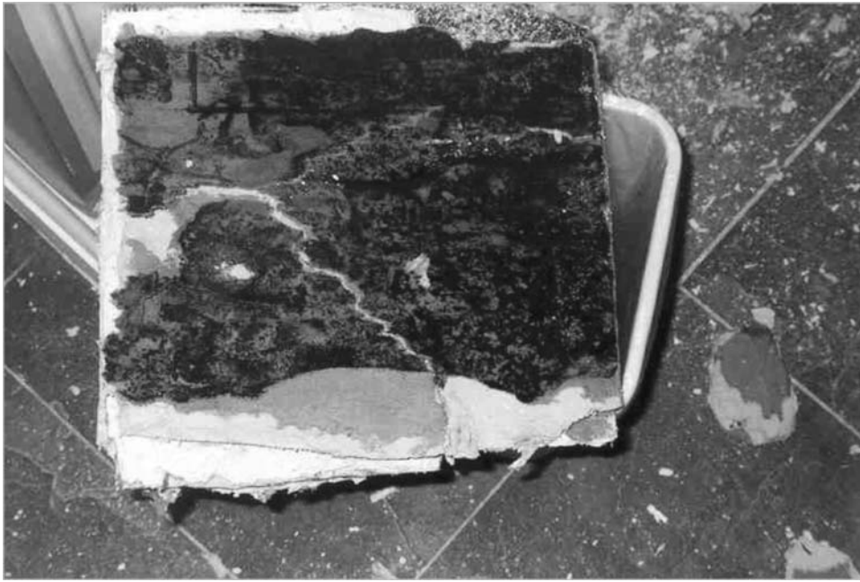
Fig. 12 Mold growth caused by infiltration in a hotel room.
