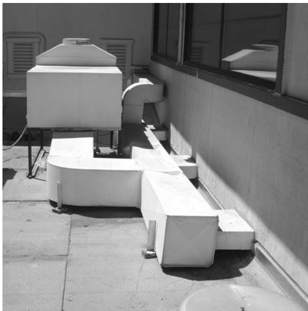
Fig. 11 A poorly installed IDEC system. The ductwork is far too restrictive to deliver the airflow needed to meet the cooling requirements of this classroom. Source: From Sacramento Municipal Utility District (see Ref. 7).
