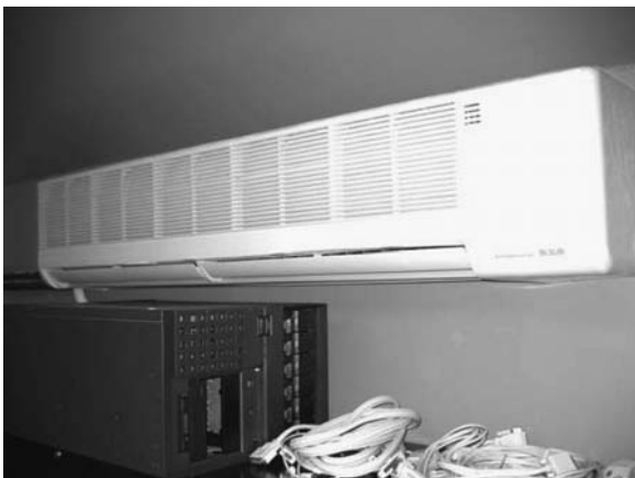
Fig. 4 Dedicated AC air-handler DX unit in computer server room.
