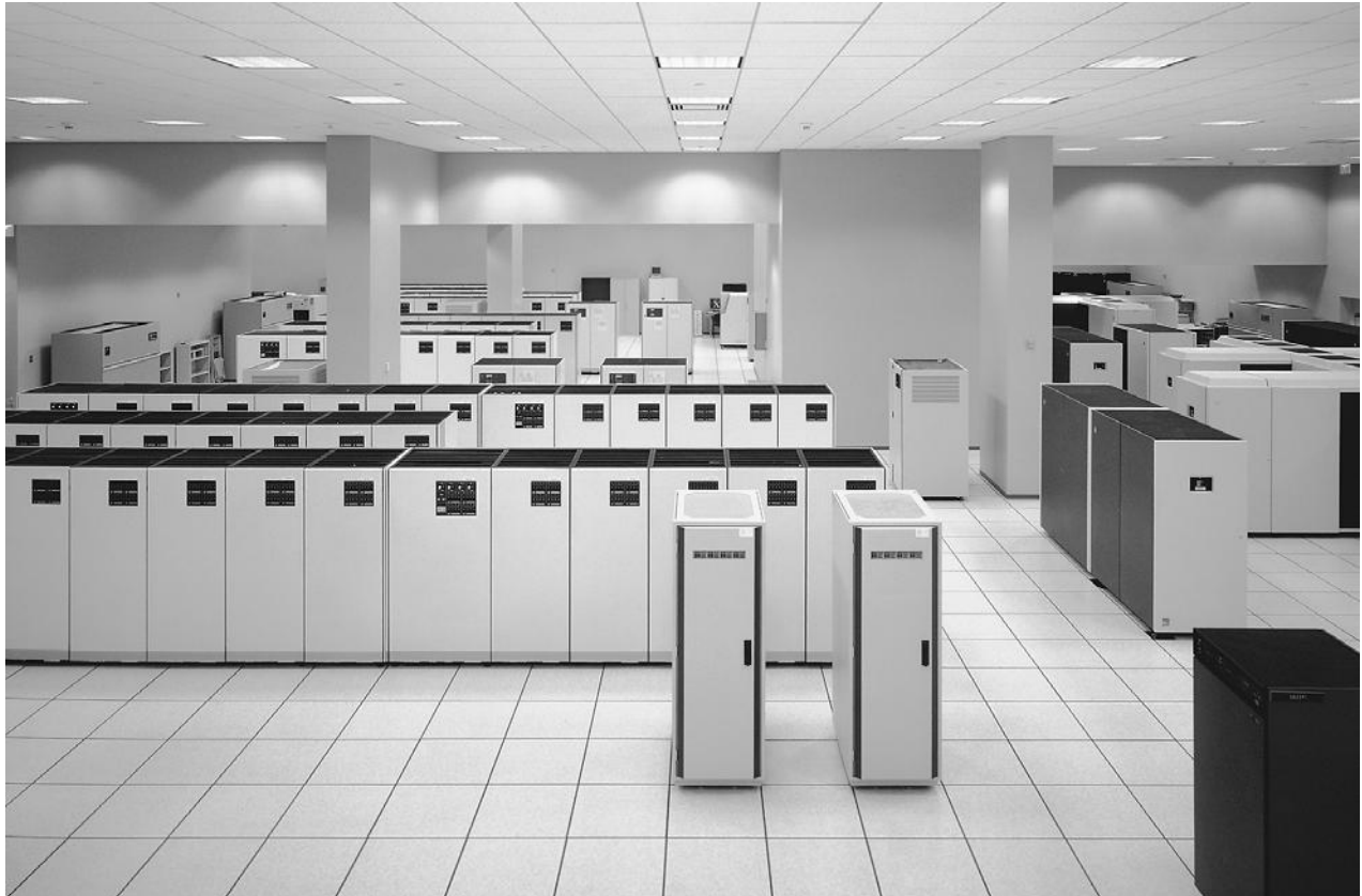
Mainframe Computer Processing Room, 2000-2003. © WES THOMPSON/CORBIS
